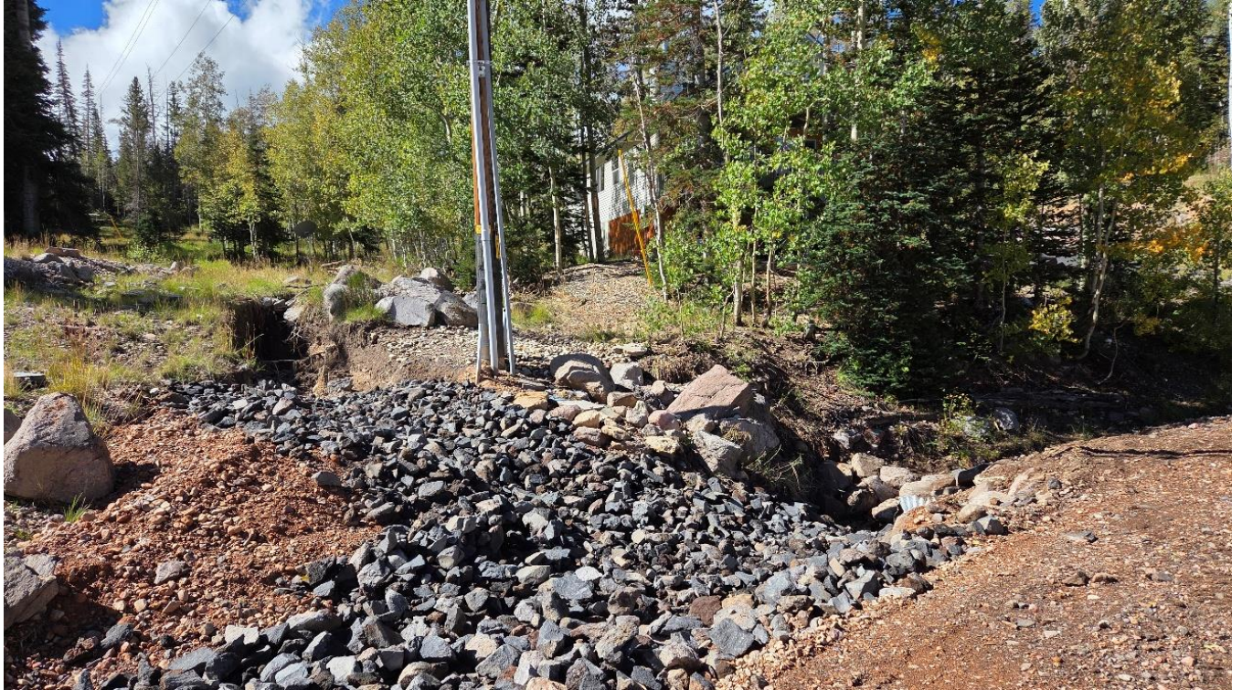
Drainage from the South side of Circle Drive, drainage from here is causing the issues
